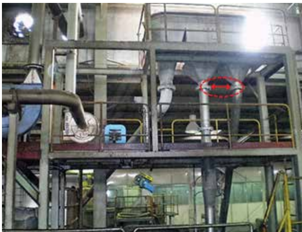
The feed and supply pipes had been incorrectly interchanged. This became visible only when inspecting the flow patterns internally.
